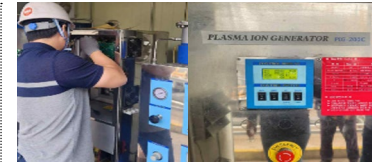
Replacement of Aging Control Panels for Dioxin Control Facilities
