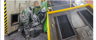
Replacement of Activated Carbon for Adsorption Towers
