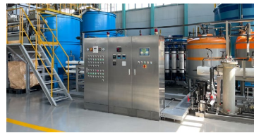
Wastewater Zero Discharge Treatment Facility
